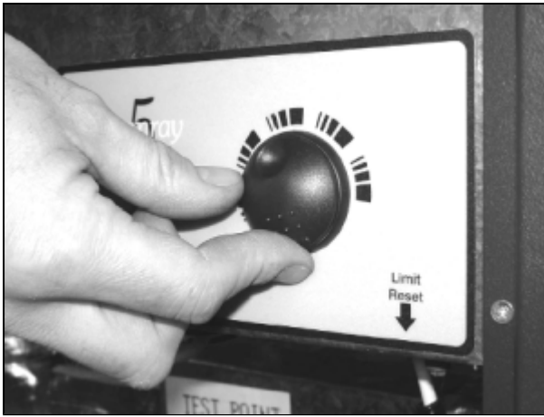
BOILER CONTROL THERMOSTAT
