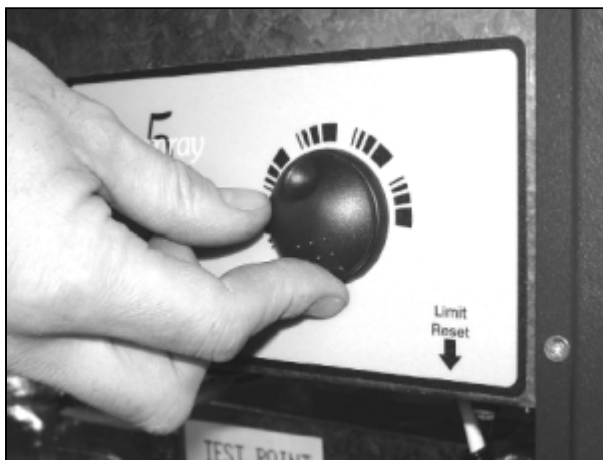
BOILER CONTROL THERMOSTAT
