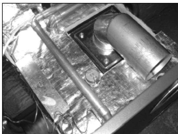
RETURN PIPE CONNECTION
