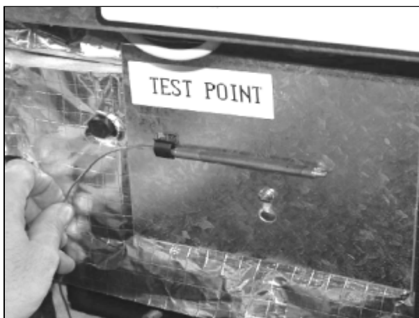
FIRE VALVE SENSOR LOCATION
