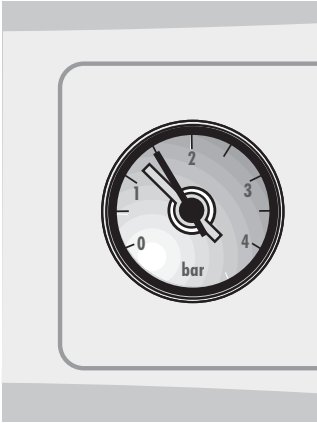
Sealed System pressure when boiler is in operation
